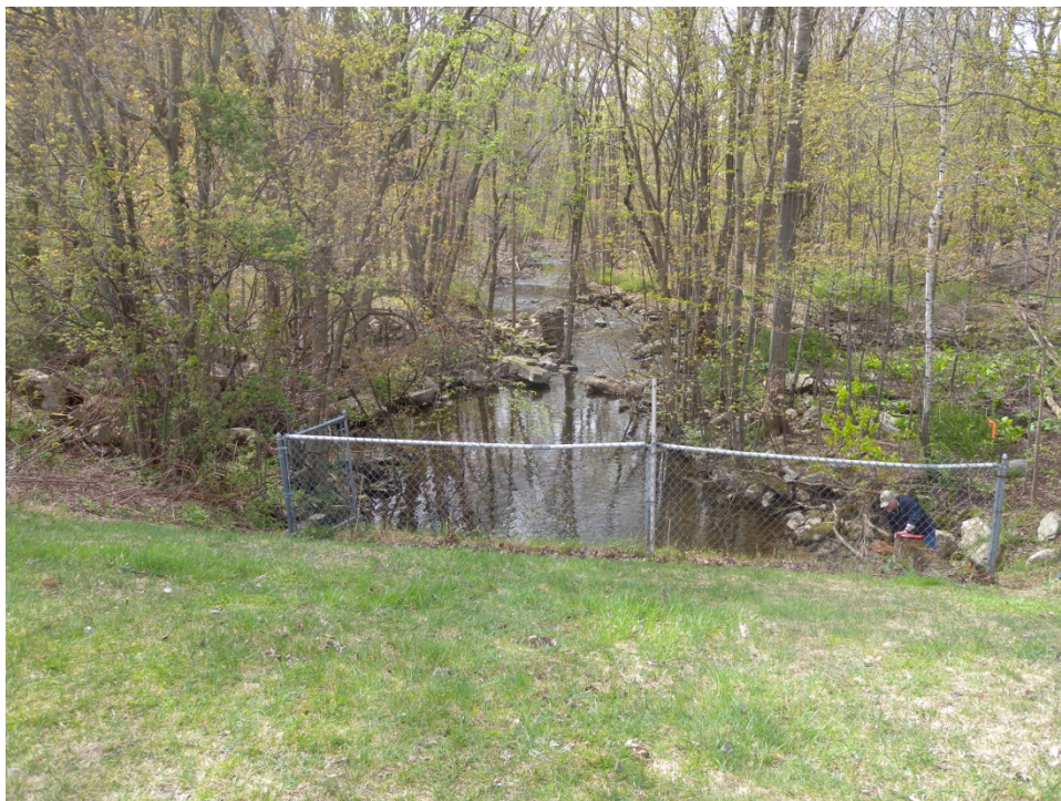
Photo 10 - EOH-07 Downstream Channel with Bridge Remnants
