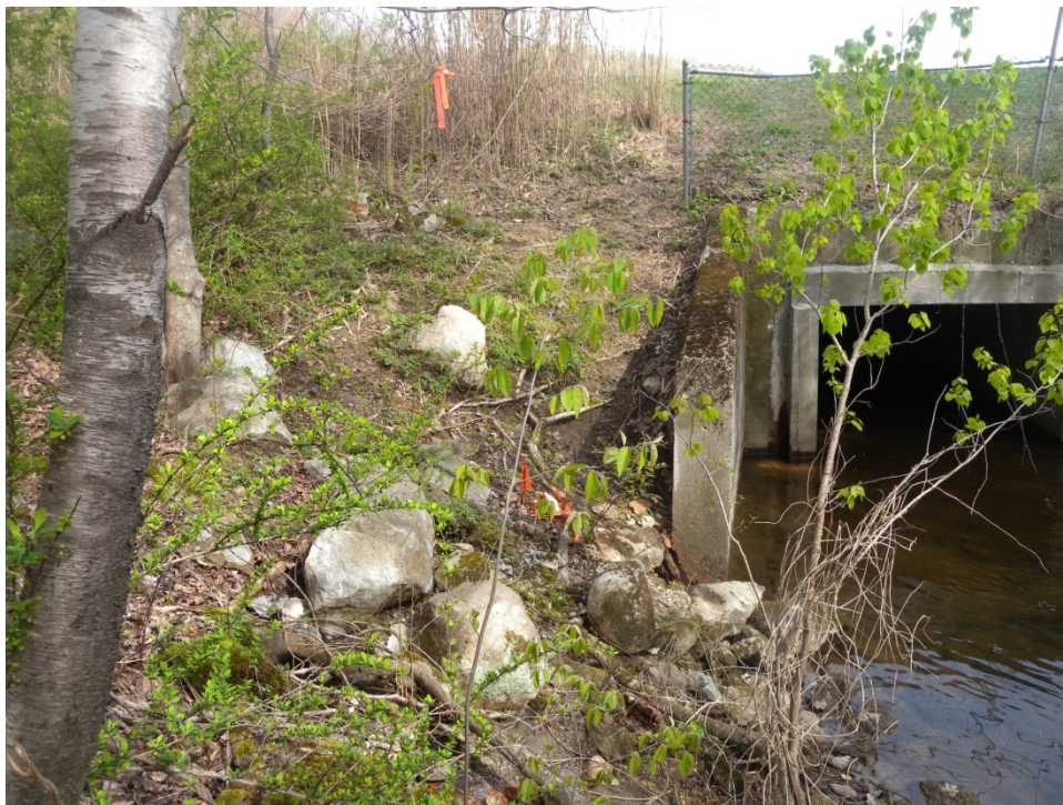
Photo 4 - EOH-07 Erosion near the Right Spillway Outlet Training Wall
