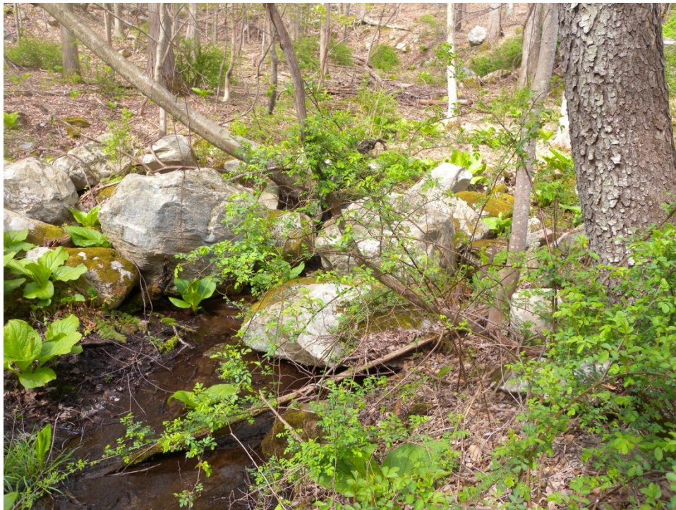
Photo 6 - EOH-07 Seepage near Right Abutment
